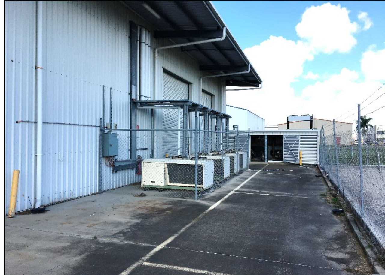
Air Cooled R404A Plant, single stage, electric defrost
