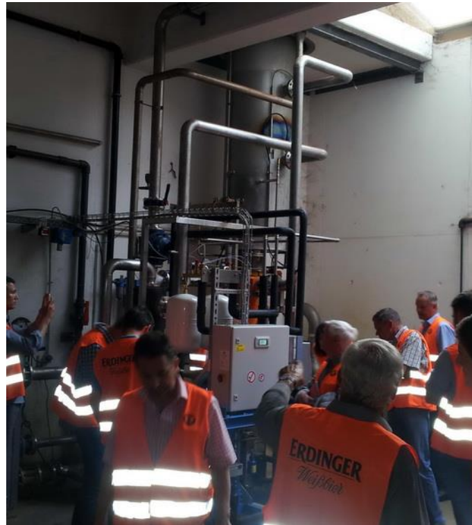
The installed chiller at DKV excursion
