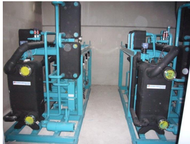
(2007) Big heat pump 6 compressors (2x 300kW) for a hard ware store in austria.
