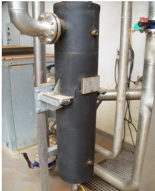
Heat exchanger for biogas
