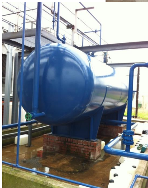
HPR Liquid Storage Vessel
