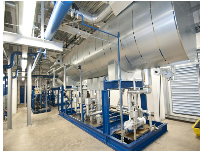
Surge Drum Vessel and Liquid Pumps
