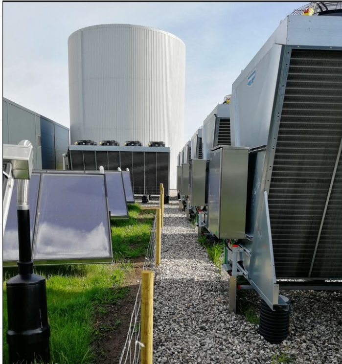
District heating facilities
