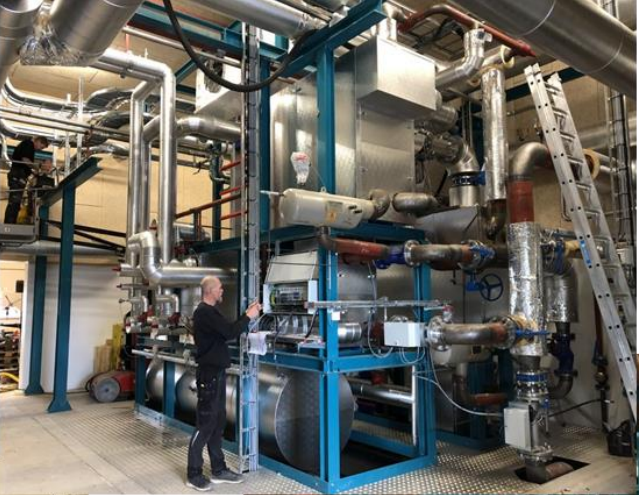
District Heating Stovring
