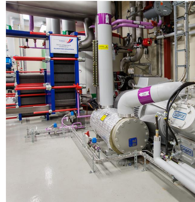
“Walking the talk“ An ammonia heat pump recovering waste heat from plate pressing is heating the main factory and head office in Lund, Sweden.
