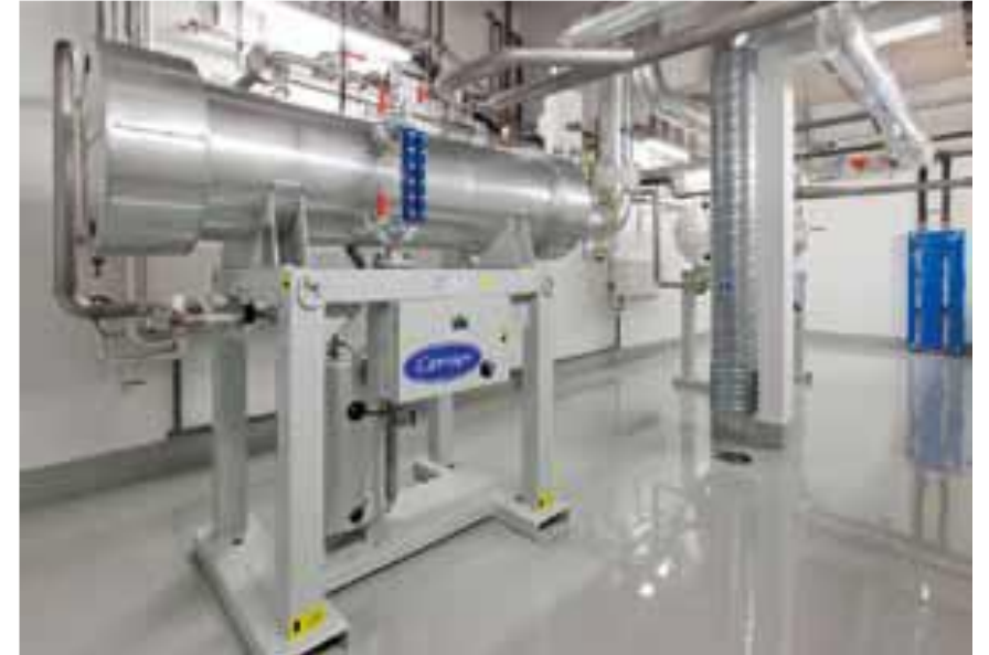
Heat exchanger (CARRIER)
