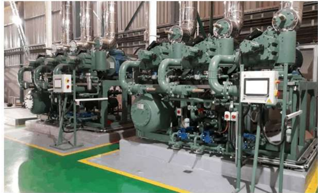
Poultry Slaughterhouse - South Africa 2 x ACP95103B-3V for Q_o=824 \text{ kW} ; t_o=-40^\circ\text{C} ; t_c=-5^\circ\text{C} 1 x ACP95103K-3V for Q_o=2.217 \text{ kW} ; t_o=-5^\circ\text{C} ; t_c+34^\circ\text{C}
