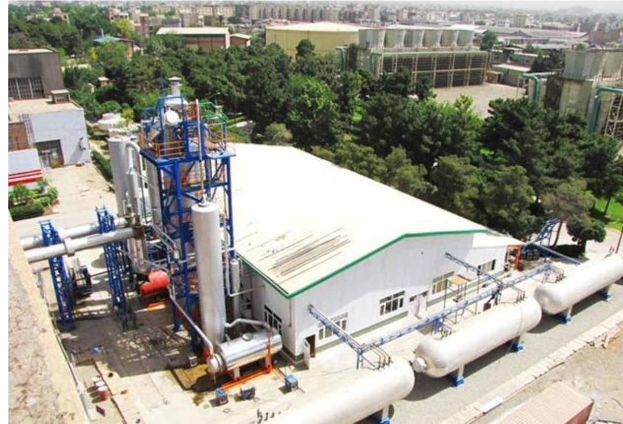
CO 2 extraction from Besat power plant
